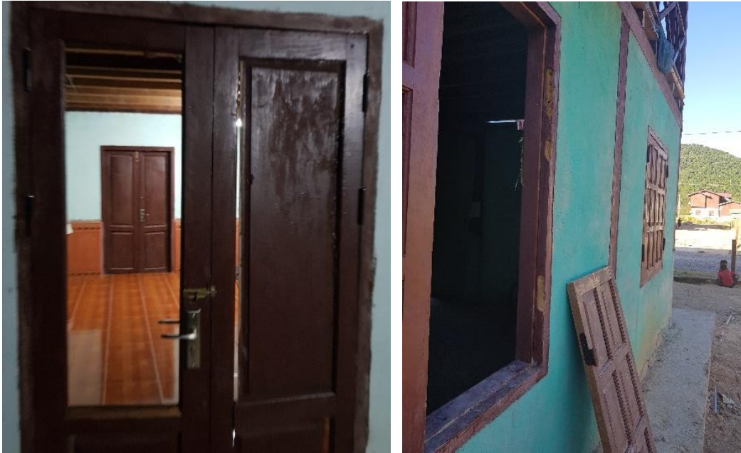
Figure 21 An example of sub-standard door and window frames in Ban Samarkkee
