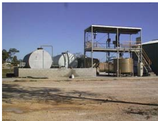
Figure 2: triple-bunded and covered chemical storage plant
