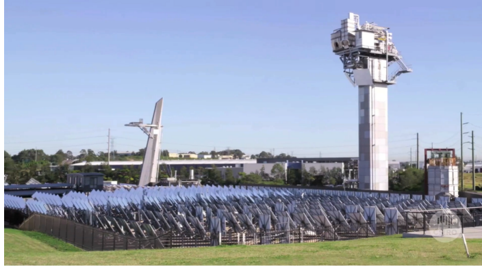
Fig. 4.3: CSIRO's heliostat field with two towers in Newcastle, NSW.
