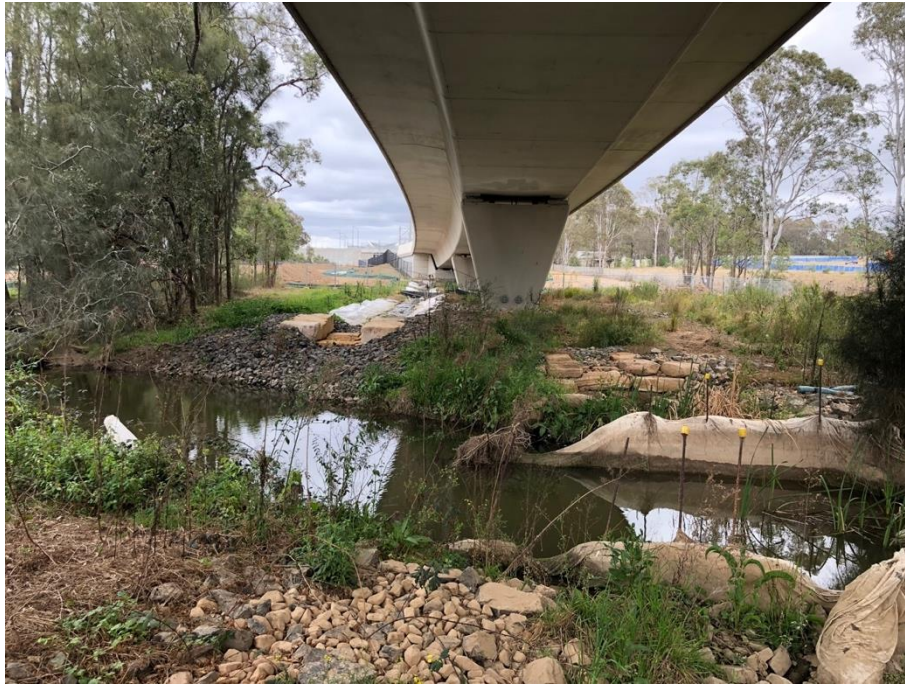
Plate 15. Disputed rehabilitation and sediment and erosion controls under a light rail project in the matter of Impregilo SpA and Salini Australia Pty Ltd (ISJV) and Sydney Metro (Sydney Metro). One part of the dispute centred around the lack of contemporaneous data and the validity of retrospective aerial photo imagery in the provision of evidence. (Photograph by author, 2019).
