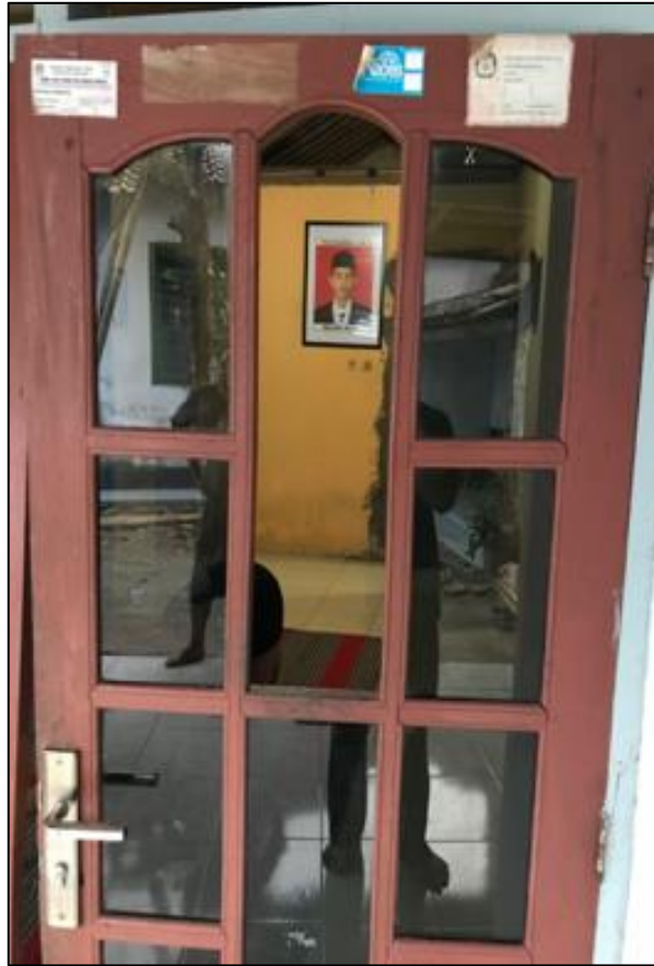
Figure 6.2: Broken door of the Tudung headman's house following damage caused by a stone
