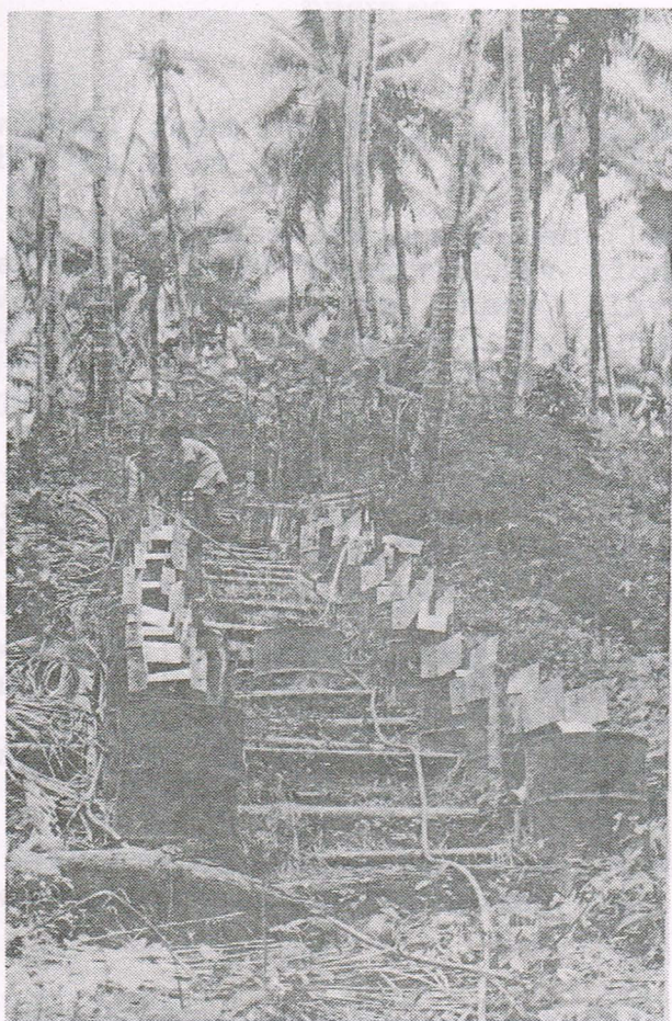
Figure 2: To collect runoff, there is a series of drums with spouts below each garden.
