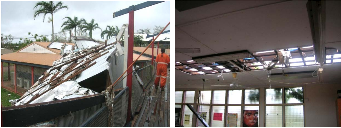
Figure 10.6: A section of roof on one of the high school buildings ripped off during Cyclone Monica and pierced through the roof of a neighbouring building, where 160 people were sheltering from the storm. Photos: courtesy of the Maningrida Emergency Response Group.
