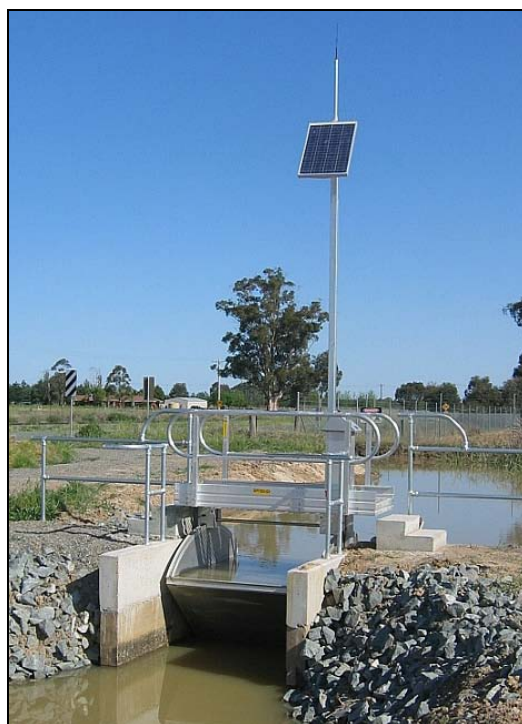
Upgraded irrigation infrastructure, Victoria, October 2008 (Photos: Catherine Gross)
