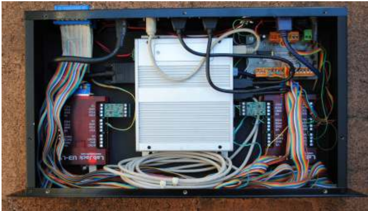
Figure 3. The new controller for the siderostats and longitudinal dispersion corrector (LDC). The unit shown is the LDC controller, which currently only uses one LJTICKDAQ. The ARK-1370 and the two LabJacks fit into a 2 unit high 19 inch rack chassis. The small printed circuit board at the upper right is the differential line receiver for the incremental shaft encoder.
