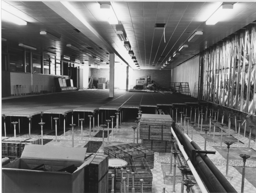
1975: Installing the false floor in the new Huxley computer room in preparation for the Univac 1100/42. (The building wasn't officially called the Leonard Huxley Building until 1987.) Photo from A Pictorial History of the CSC.
