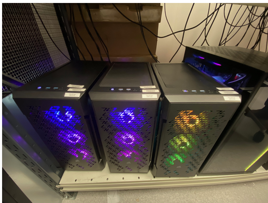
Gaming machines whose GPUs are doing important computation for the Australian Centre for Robotic Vision. They're located in a small server room in Brian Anderson Building along with dozens of other GPU-festooned research servers. Photo: David Hawking
