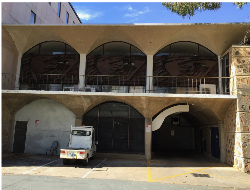
The basement “Elephant Stables” under the Menzies Library which housed the first Univac installation.
