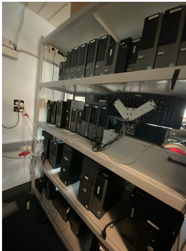
The small server room on Level 2 of the CS&IT Building which houses the file servers and some image servers for the student labs, as well as some other production servers. Photo: David Hawking
