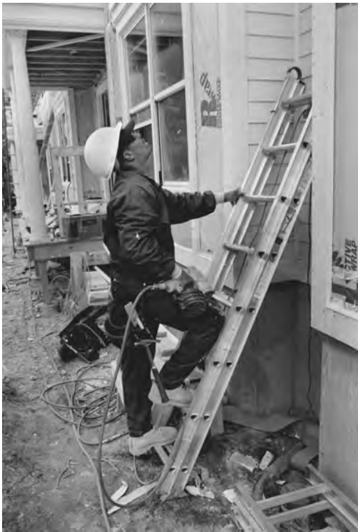
Figure 15-4. Example of poor housekeeping on a construction site. Numerous cords and debris create a potential tripping hazard for workers. (Photograph by Earl Dotter.)
