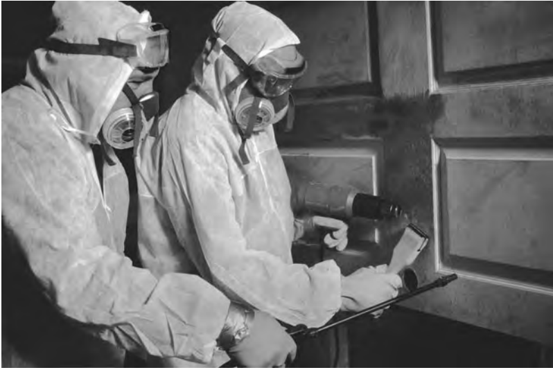
Figure 1-6. Lead-based paint in many older homes still represents a serious health hazard to many young children. This photograph depicts a lead abatement worker with personal protective equipment. Workers performing lead abatement must be trained and certified, and they must carefully adhere to safe practice standards. (Photograph by Earl Dotter.)
