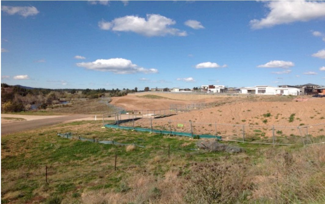
Figure 7.16 Sediment control and fence along the edge between Coombs and the river
