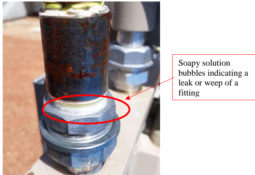
Figure 5. Leak location with “Soapy Solution”
