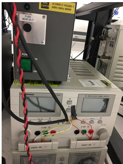
Fig. A.3 Below the optical table, from top to bottom are polygon driver power supply, PMT amplifier power supply and galvo driver power supply.
