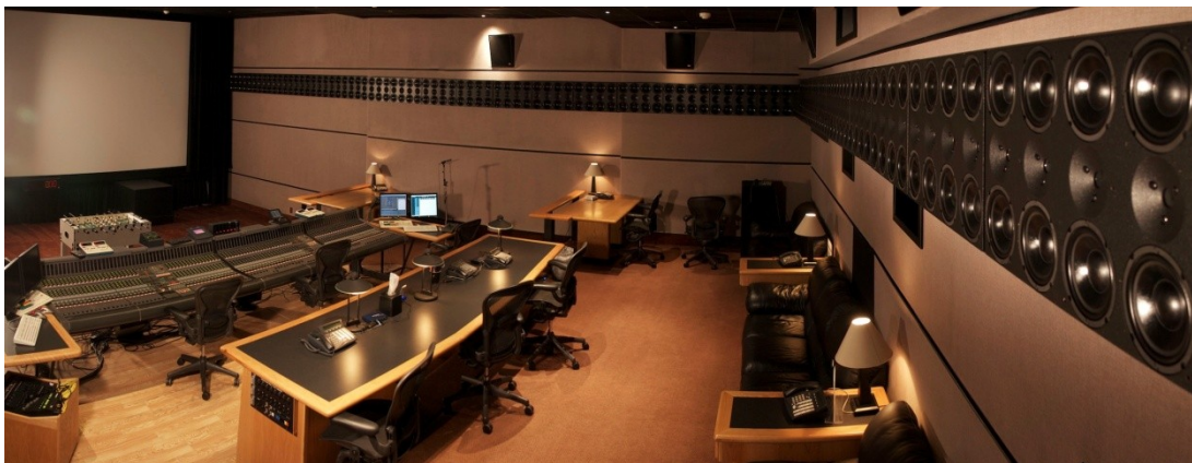
Figure 6: IOSONO Sound installation Todd-AO, Burbank, USA 79
