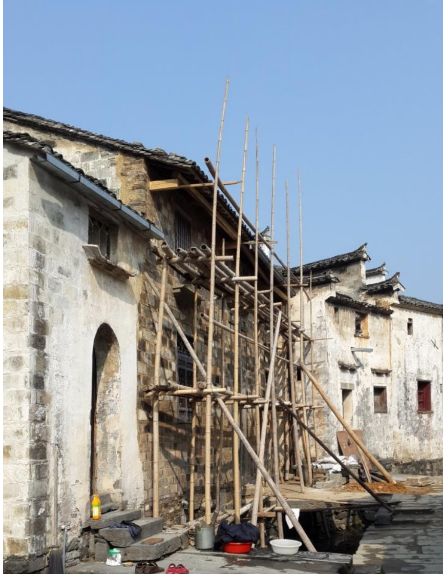
Fig. 9.4 XD083 was repairing his old house (photo by Rouran Zhang)
