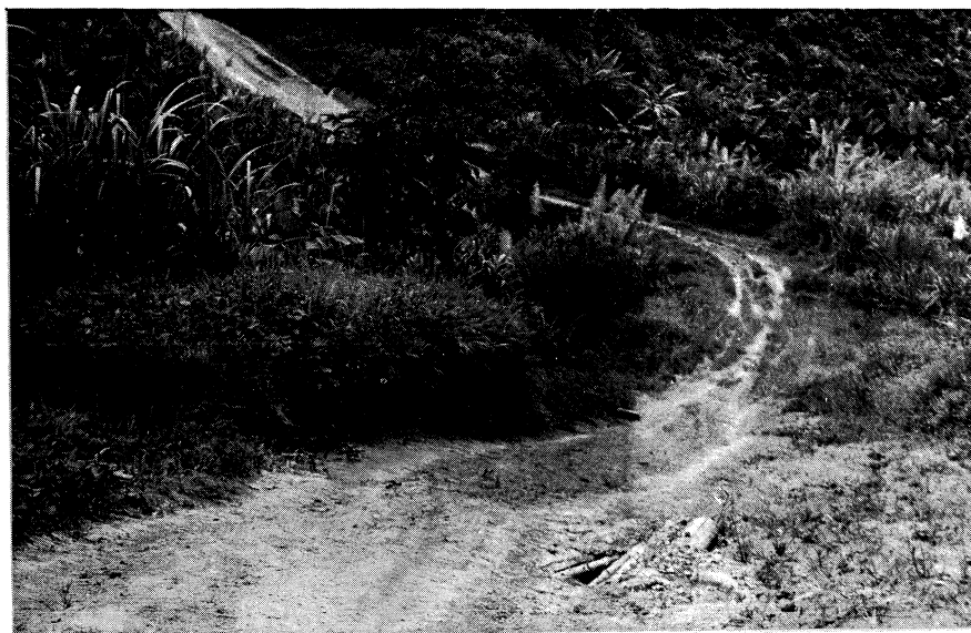
The 'Kombio Road', south of Yasip. Typical unsurfaced side road. Clay surface, poor alignment, timber culverts, insufficient drainage, numerous swampy patches. Virtually impassable when wet.
